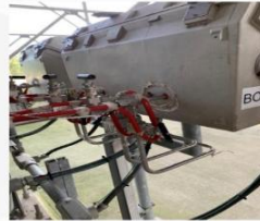
Enhanced Equipment Heat Tracing
